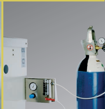
Control panel with indicator Installed on mixer
